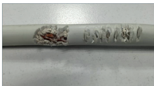
Example of mouse bite marks in the cable sheath Source: Pepperl+Fuchs
