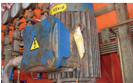
Example of corrosion caused by chemicals Source: thuba AG
